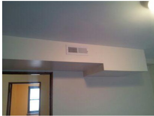
Newly Installed Heating Ducts
